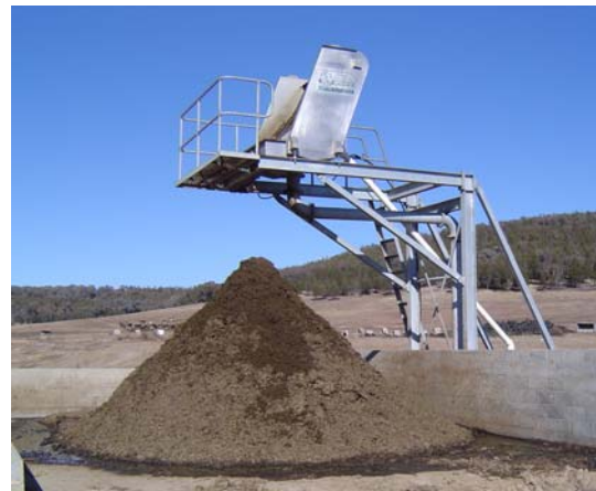
A “Wedge-Wire” screen in operation
