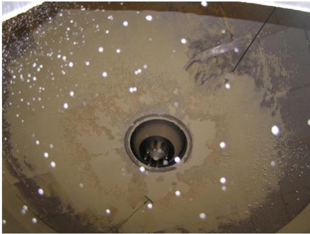
Fouling of dryers
