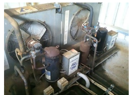
Figure 3 Software with simple graphics to view energy use on each circuit
